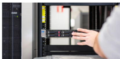
Section 7 Step 5—Future-proof your infrastructure
